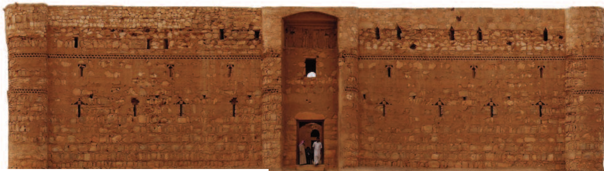
Qasr Kharana. Southern Façade. Scale 1/50. November 2009 Spanish Archeological Mission/ Institute Juan de Herrera Survey Director: Dr. Ignacio Arce Photo Rectification: Mr. Ignacio Moscoso
